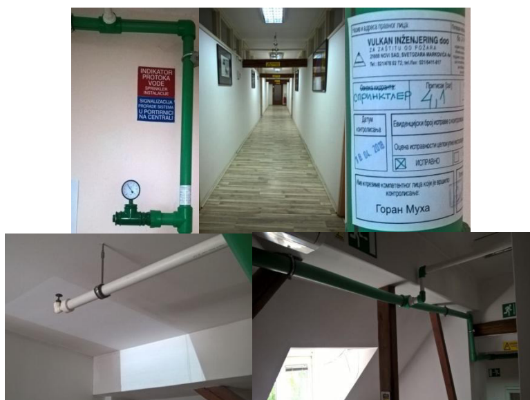
Figure 5 – Sprinkler network with the card for regular maintenance; source: author (photographed on 28 th May, 2018)
