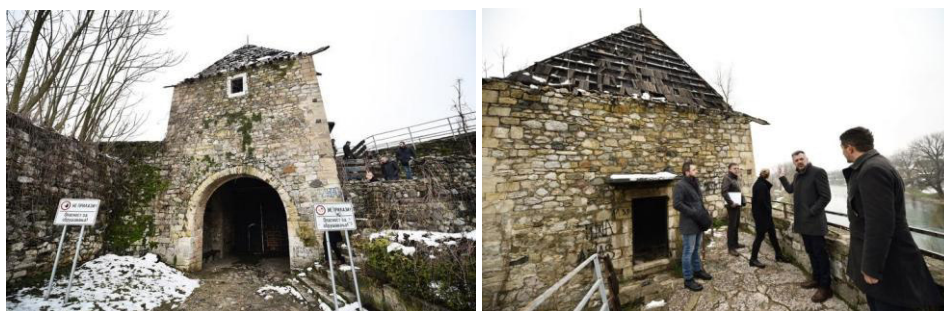
Figure 2 – Kastel Fortress: damages to tower 1 after the fire
