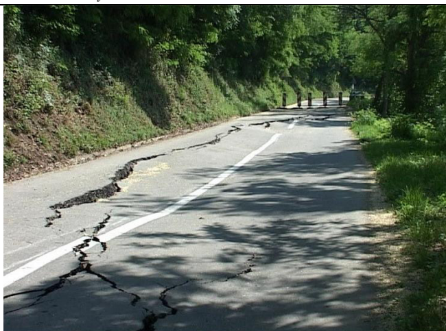
Figure 1 – Head cracks and denivelation of the terrain on the road, as clear indicators of terrain instability. [7]
