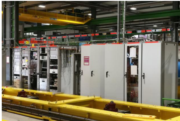
Figure 1 - Open/closed cabinets + racks in a row – picture from one of CERN facilities
