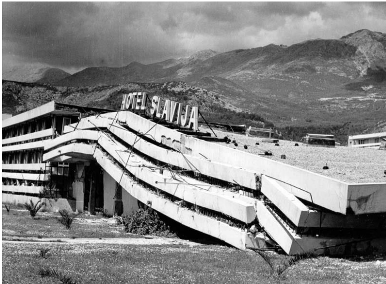
Figure 2. Soft-story collapse, followed by the collapse of the whole structure of Hotel “Slavija” in Budva after the Montenegro earthquake in 1979 (R. McGuire, U.S. Geological Survey, 1979)
