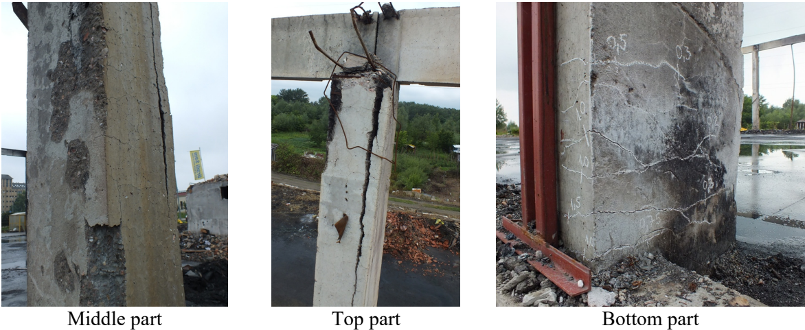
Fig. 26. Characteristic fire damages of RC columns
