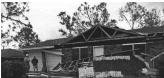
Fig. 4a. Porch overhang collapse due to lack of anchorage for support column/post (Van de Lindt et al. 2007)
