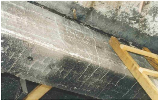
Fig. 8. Crazing – mesh like cracks
