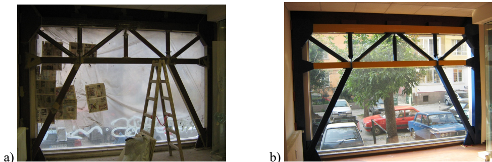
Fig.5a,b Steel-truss frame system developed for strengthening of reinforced concrete frames with infills, as well as to masonry structures
