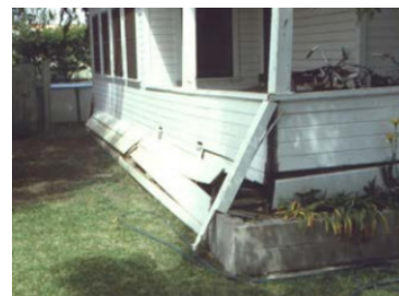
Fig. 4b. The porch in front of this house has collapsed due to inadequate bracing, Whittier earthquake, 1987 (Arnold 2002)
