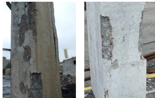
Fig. 4. Corner spalling and corner cracks along main reinforcement
