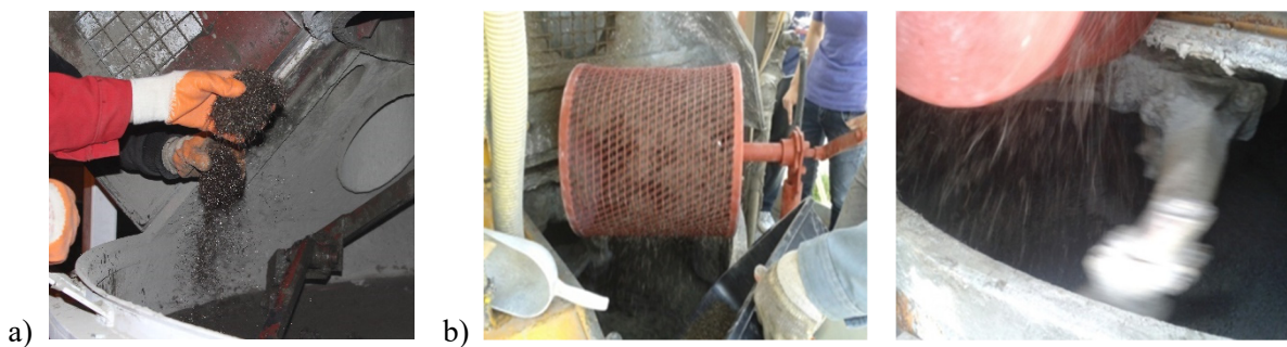
Fig. 4. a) Manual addition of fibres to concrete batching plant; b) Drum for the addition of the fibres
