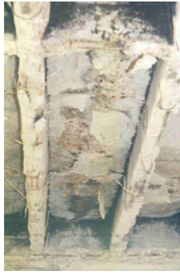
Fig. 19. Influence of defects on fire damages degree in pan joist floor system
