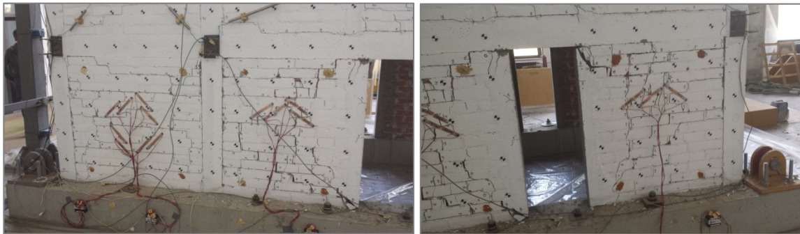
Fig. 13 Damage to the infill of the MODEL 2
