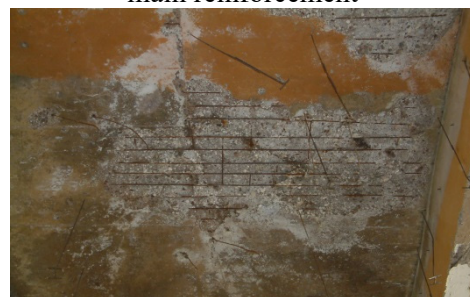
Fig. 6. Sloughing off spalling (slab)
