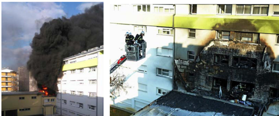
Fig. 1. a) student dormitory during fire b) the façade after the fire was extinguished [3,4]
