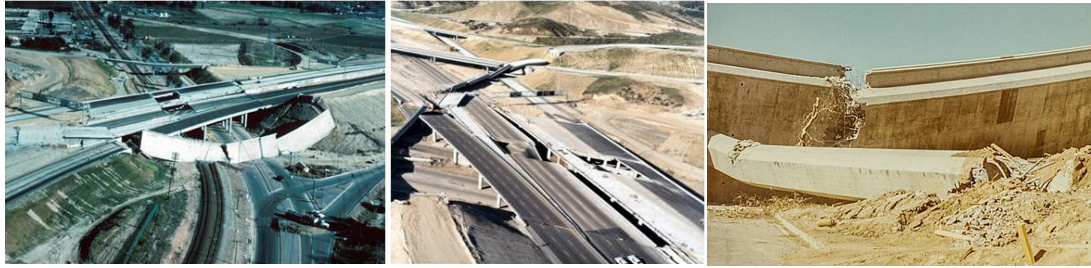
Fig. 8. Failure of I-210 overpass to I-5 south with column failure
