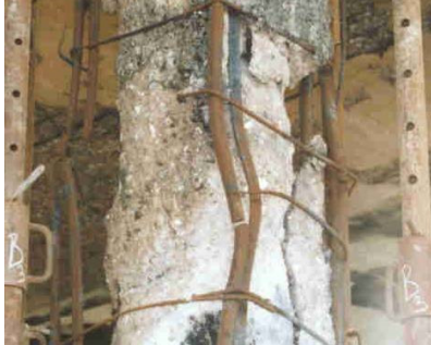
Fig. 10. Plastic deformations and breaking off of bars
