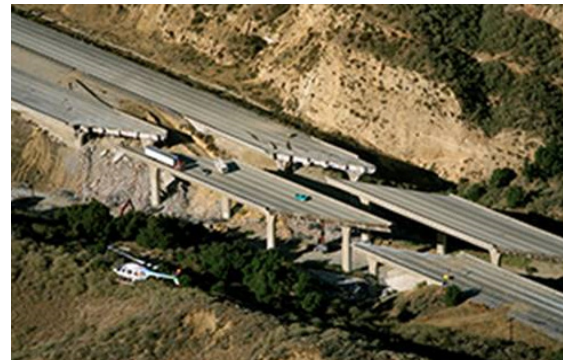
Fig. 7. I-5 Newhall bridge failure near SR14
