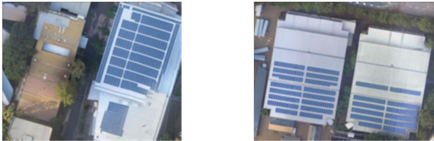
Fig. 6. Aerial views of partially completed solar installation at University of Queensland (Pearce 2017)
