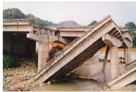
Fig. 6b. Girder unseating in the 1999 Chi-Chi Earthquake Taiwan (Moehle and Eberhard 2000)
