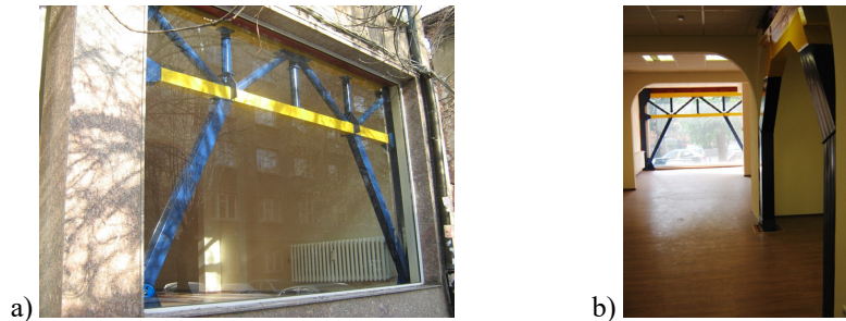
Fig.1a,b View outside and inside on the steel frame in residential building
