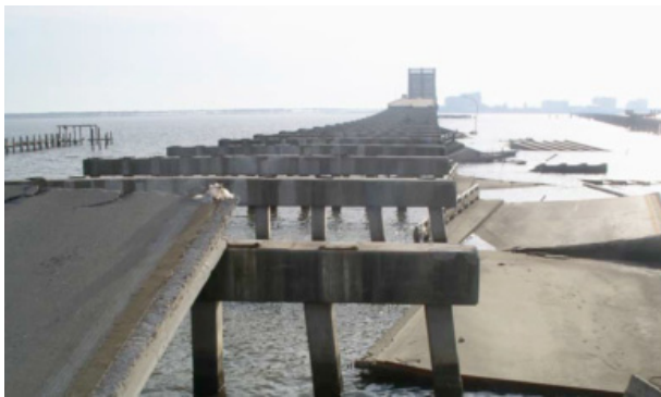
Fig. 6a. Span unseating due to storm surge-induced loading on US-90 Biloxi-Ocean Springs Bridge (Padgett et al. 2008)
