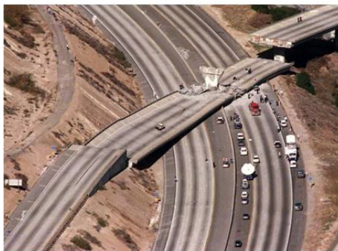
Fig. 6. SR14 ramp collapsed onto I-5
