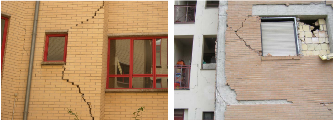
Fig.1 Damages on infill
