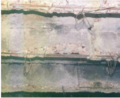
Fig. 15. Typical damages of pan joist floor system due to fire
