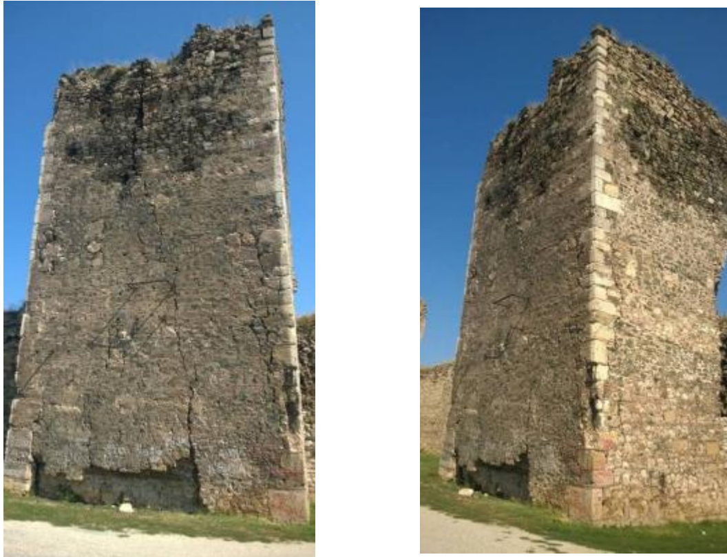
Fig. 5. Degradation of building elements of Tower 11
