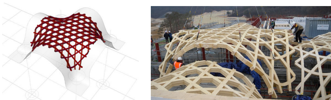
Fig. 5. The Yeosu golf clubhouse in Republic of Korea under construction; digital simulation of the roof and a part of the roof during assembly
